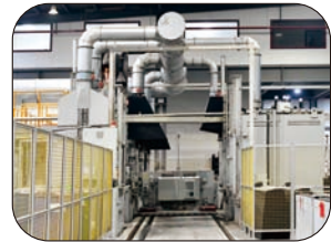
IPSEN Carburising Equipment (Germany-made)
