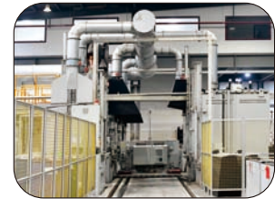
IPSEN Carburising Equipment (Germany-made)
